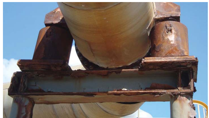
NON PT&P Painted Support 8 Years In-Service in Louisiana
