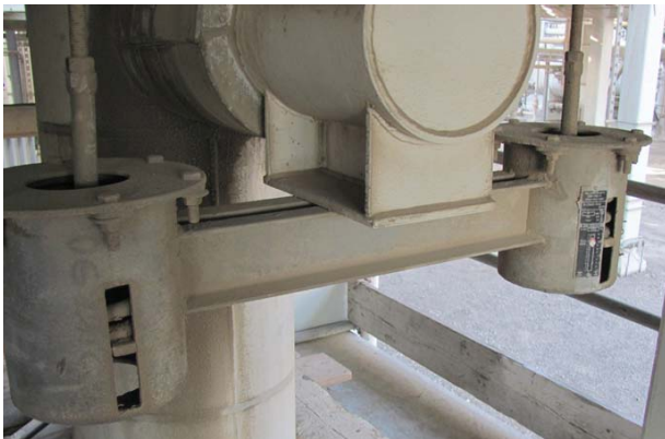
PT&P Hot-dipped Galvanized Support 25 Years In-Service
